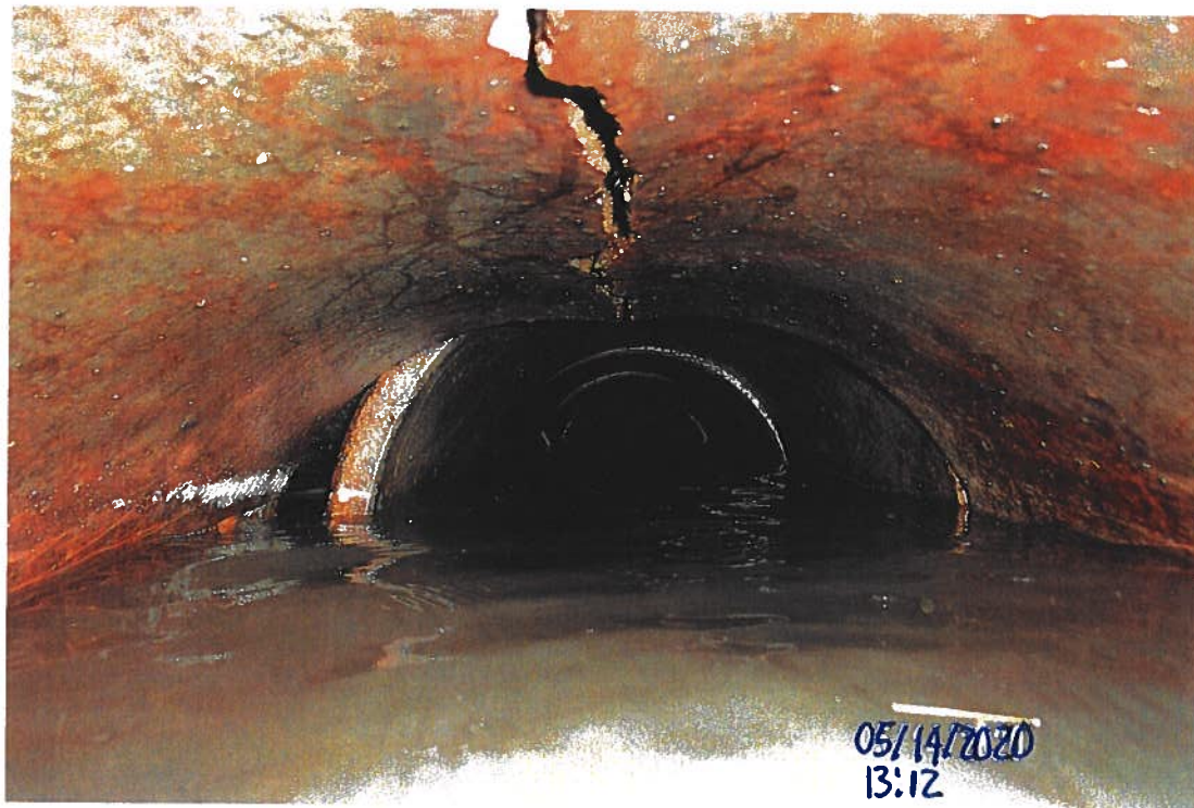
PICTURE # 3552 IS LOOKING SE SHOWING 1ST SECTION OF CLAY TILE WITH LONGITUDINAL CRACKS AND CAVING DOWN DOWNSTREAM FROM CPS# 139 WITH REST OF SECTIONS OF TILE NOT LOOKING TOO BAD
