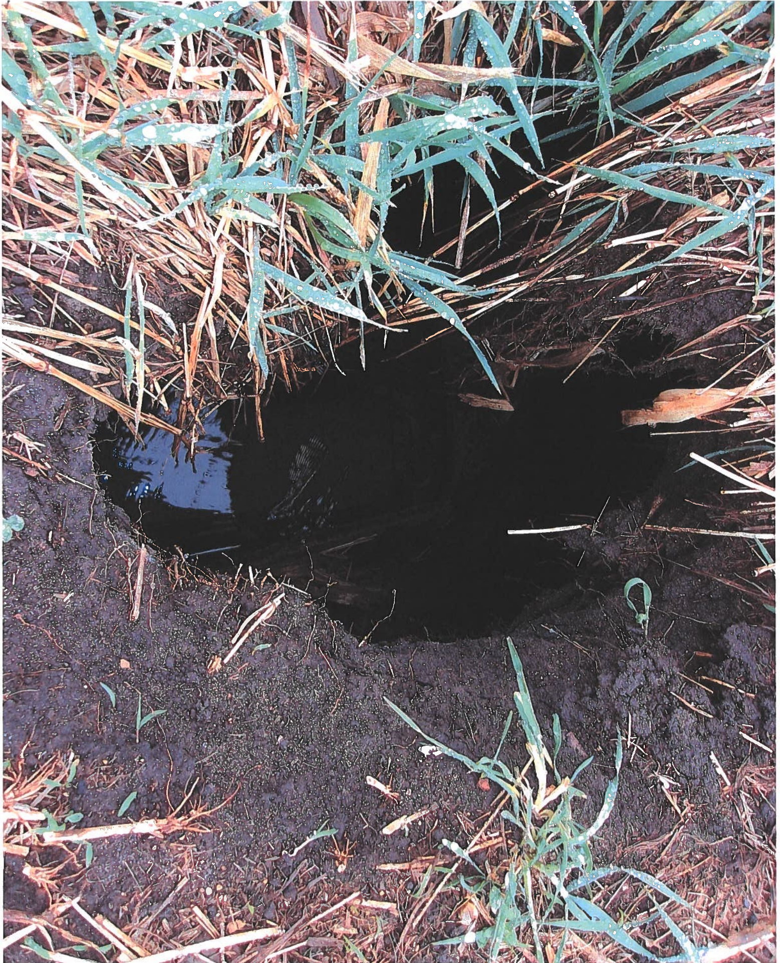
Collapsed Clay Tine
