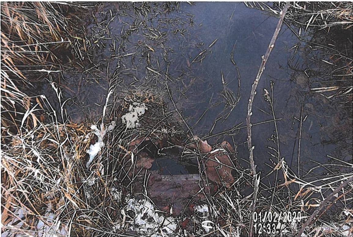
PICT# 2619 TOP VIEW OF MANGLED 30" CMP OUTLET ON N SIDE OF RR ACCESS DRIVE
